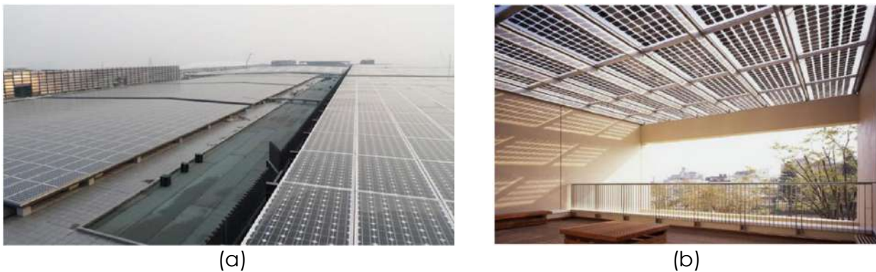
Figure 4: Example PV installations: (a) BAPV and (b) BIPV [9]
